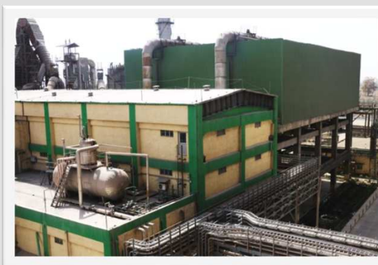
Waste Heat Recovery System
