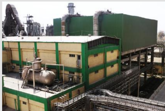
Waste Heat Recovery System
